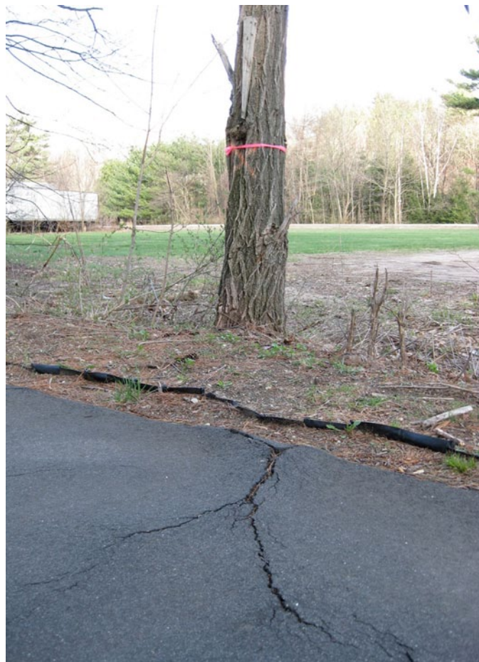
Tree root damage Manhan Rail Trail, MA.
