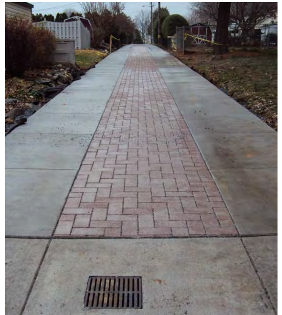
Alley 148 was redesigned to feature porous pavers atop an aggregate (gravel) infiltration trench.
